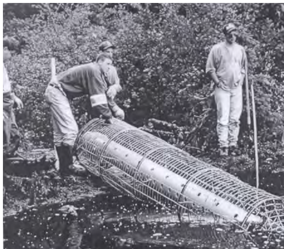
Figure 5. Clemson leveler intake pipe
