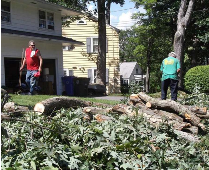
Figure III.8: Storm Damage repairs in Torrington Area after Heavy Rain, Winds, and Power Outages
